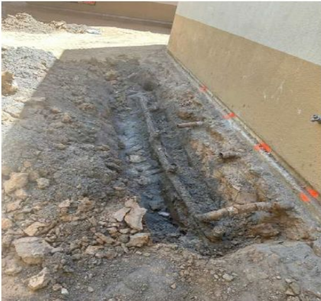
2" drains from sinks
